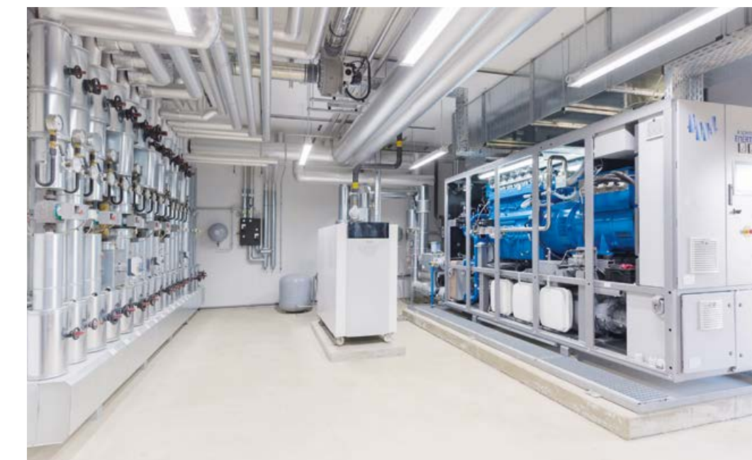
// 140 kW CHP in an educational institute in Germany
