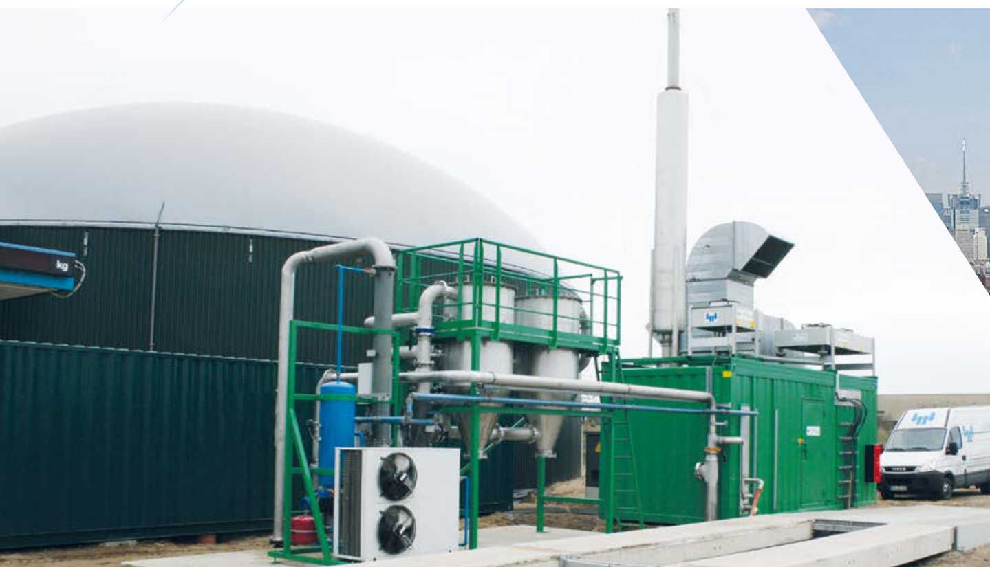
// 400 kW CHP in a Biogas plant with gas cleaning system in Germany
